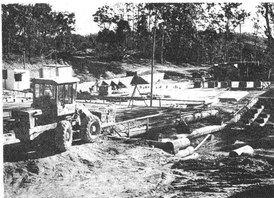
BUILDING SITE — Construction of the new administration building of the Work in Australia in Burleigh Heads is in its fourth month. Left photo: Construction progresses at the main reception area and church-
